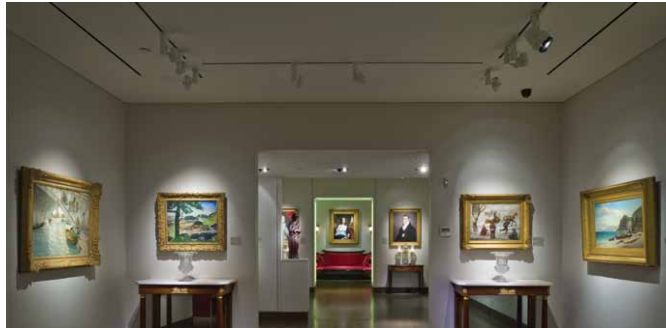
Old PAR38 halogen track heads from the previous space combine with LED and MR16 track heads, slicing energy use in half. The design team got creative and counted the walls as “merchandise” space in this retail-zoned building, in order to grab more watts.
